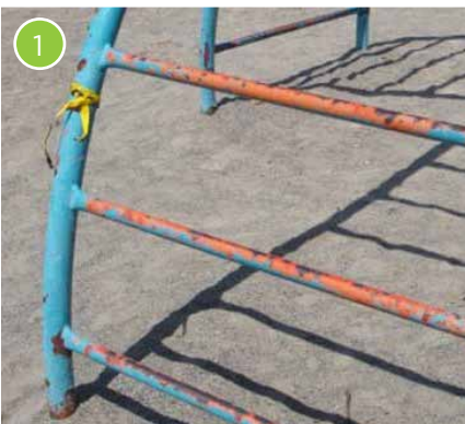
Chipped paint on this equipment should be addressed and repainted.
