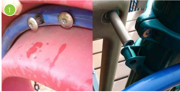
1 This bolt is loose and should be tightened or replaced.
